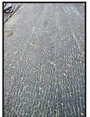
The photo here is of Malavya Avenue in Thiruvanniyur, where the road was dug up last month and is still awaiting tarring. Vehicle users find it a Herculean task to drive their vehicles here. We request that the Greater Chennai Corporation (GCC) relay the road without any further delay. N . M a h a d e v a n , Vannanthurai.
